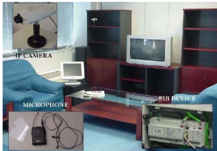
Figure 1: Snapshot of the living room and details of some system parts and components: EIB domotic control bus, IP camera and wearable microphone for input data, dynamic photo-frame and multimedia network of speakers and TV set.
